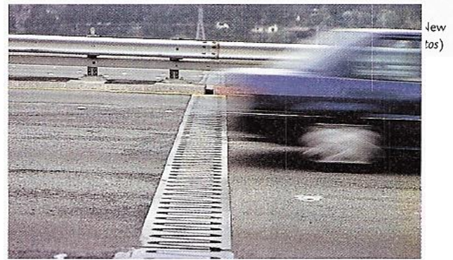
This gap in the roadway of a bridge is called an expansion joint; it allows the bridge to expand and contract. (Was this photo taken on a warm or a cold day?)
